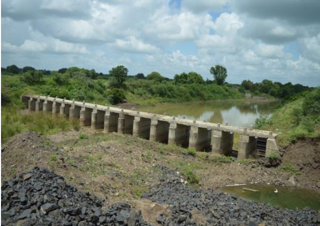
A newly constructed KT Weir on Bobhati River near Hadgav Project Village
