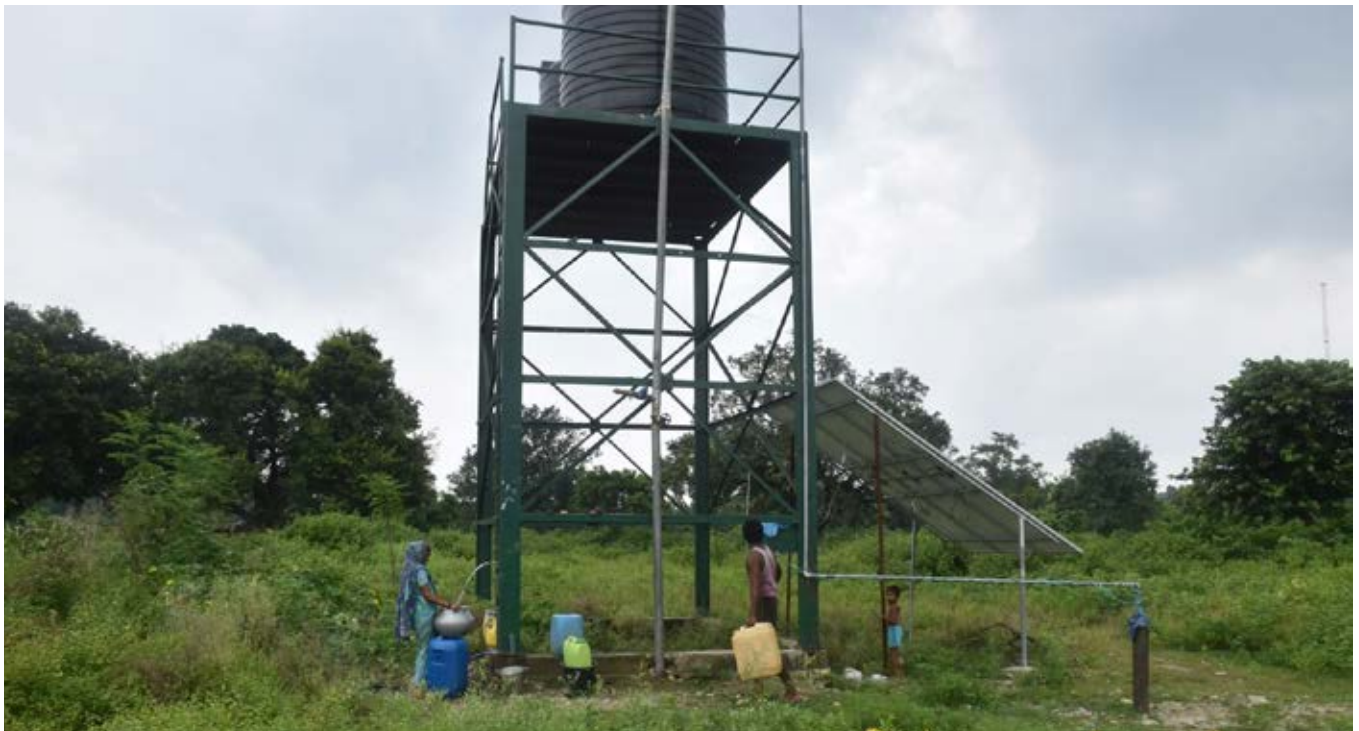
(The overhead water tank in the Bhiknathodi village under the 'Har Ghar Nal Ka Jal' popularly known as Nal-Jal Scheme of the State Government: Photo taken during the field visits made on 31.08.2020)
