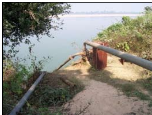
A view of irrigation point managed by Water User Association/LAWP of village Rekula of Ramial sub-basin
