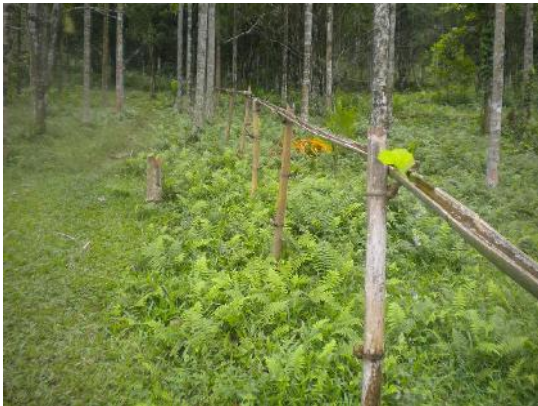
P12: Split bamboo Conveyance system for Drinking water in Sommeffre
