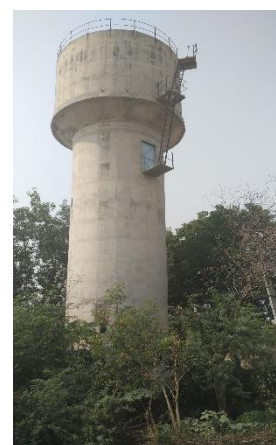
Exhibit 9: Public water supply tank
