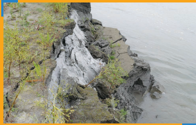
Riverbank erosion in the study area
