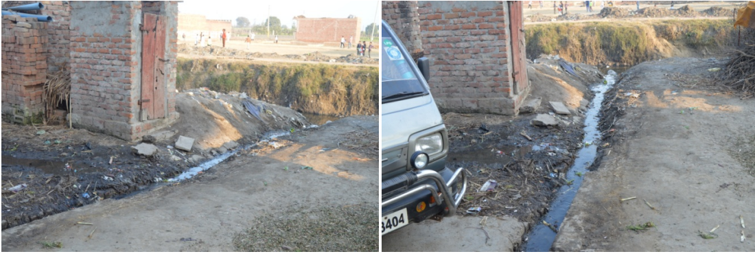
Open Drains and Waste Disposed
