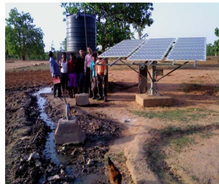
Water lifting by using Photovoltaic Water Pumps
